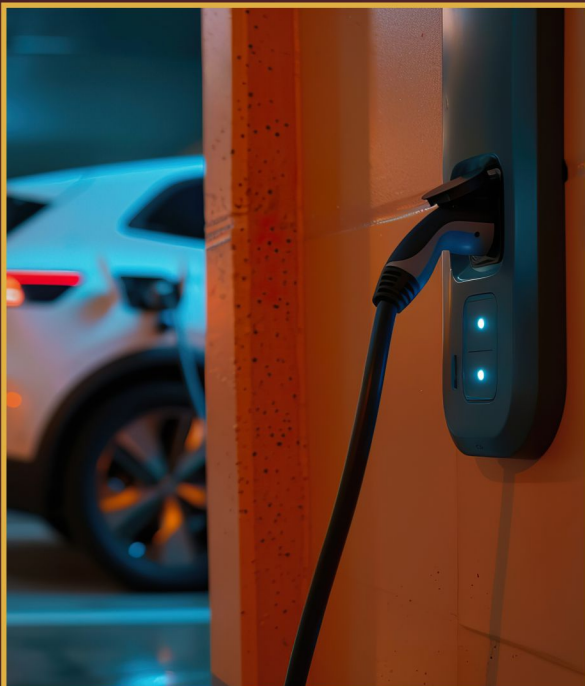
EV Charging Stations Future-ready infrastructure
